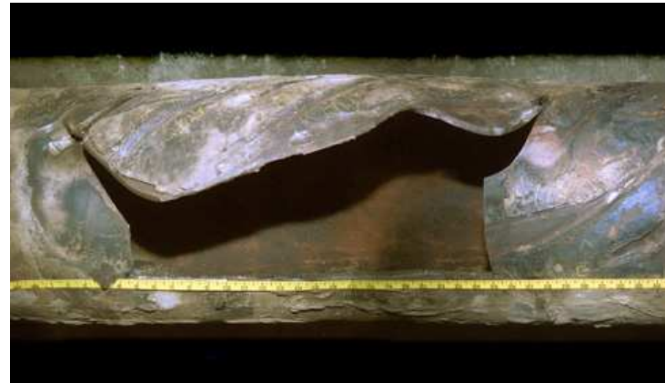
Fractured gasoline line—undetected damage
